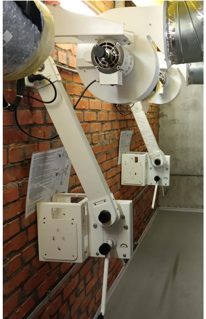
Shelter high pressure electric blower with manual backup
